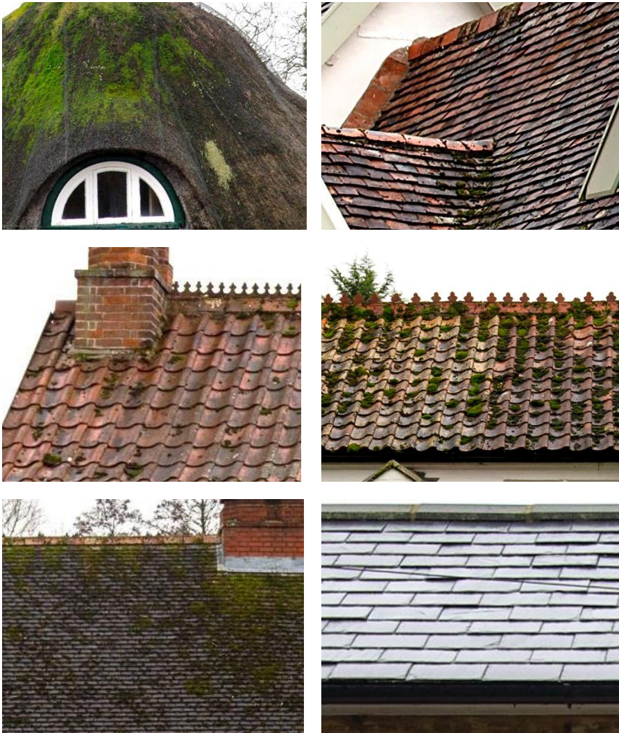
Examples of roof materials such as: thatch, clay and slate pantile, clay pantile.
